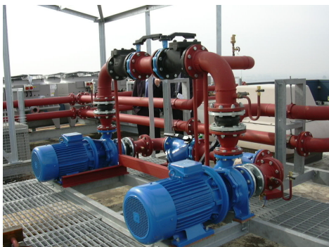
One of Westway Cooling's installations
